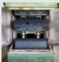
Bucket elevator boot
