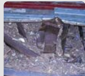
Missing predetermined breaking point
