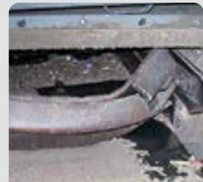
Missing predetermined breaking point
