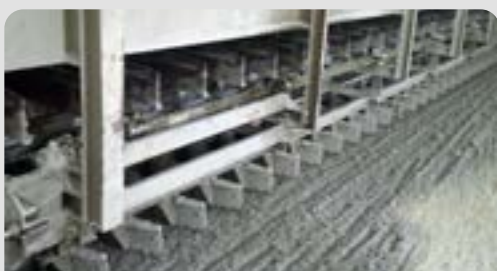
Portal scraper for granulated blast furnace slag
